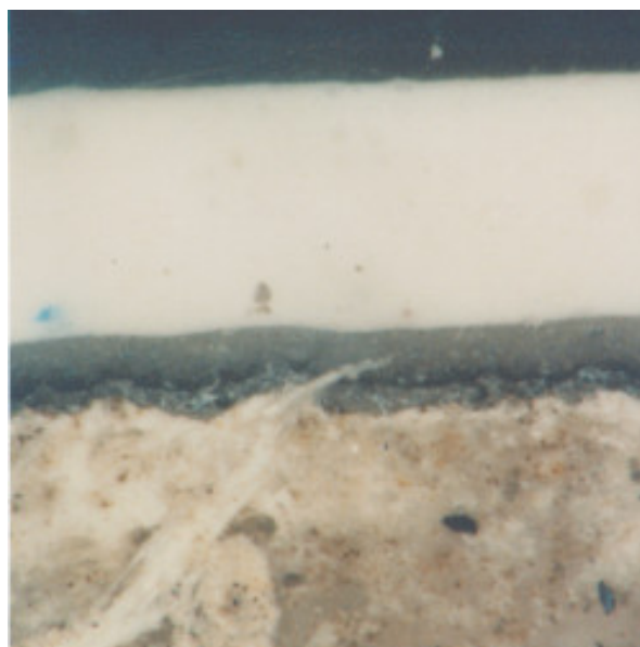
This picture highlights both the penetration of the primer into the asbestos cement as well as the efficiency of the encapsulation of the asbestos fibres which is already guaranteed by the primer
