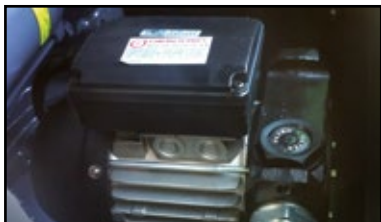
AUTOMATIC-MANUAL FUEL TRANSFER PUMP.
