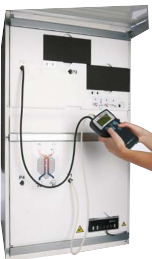
Pressure outlet on HCV
